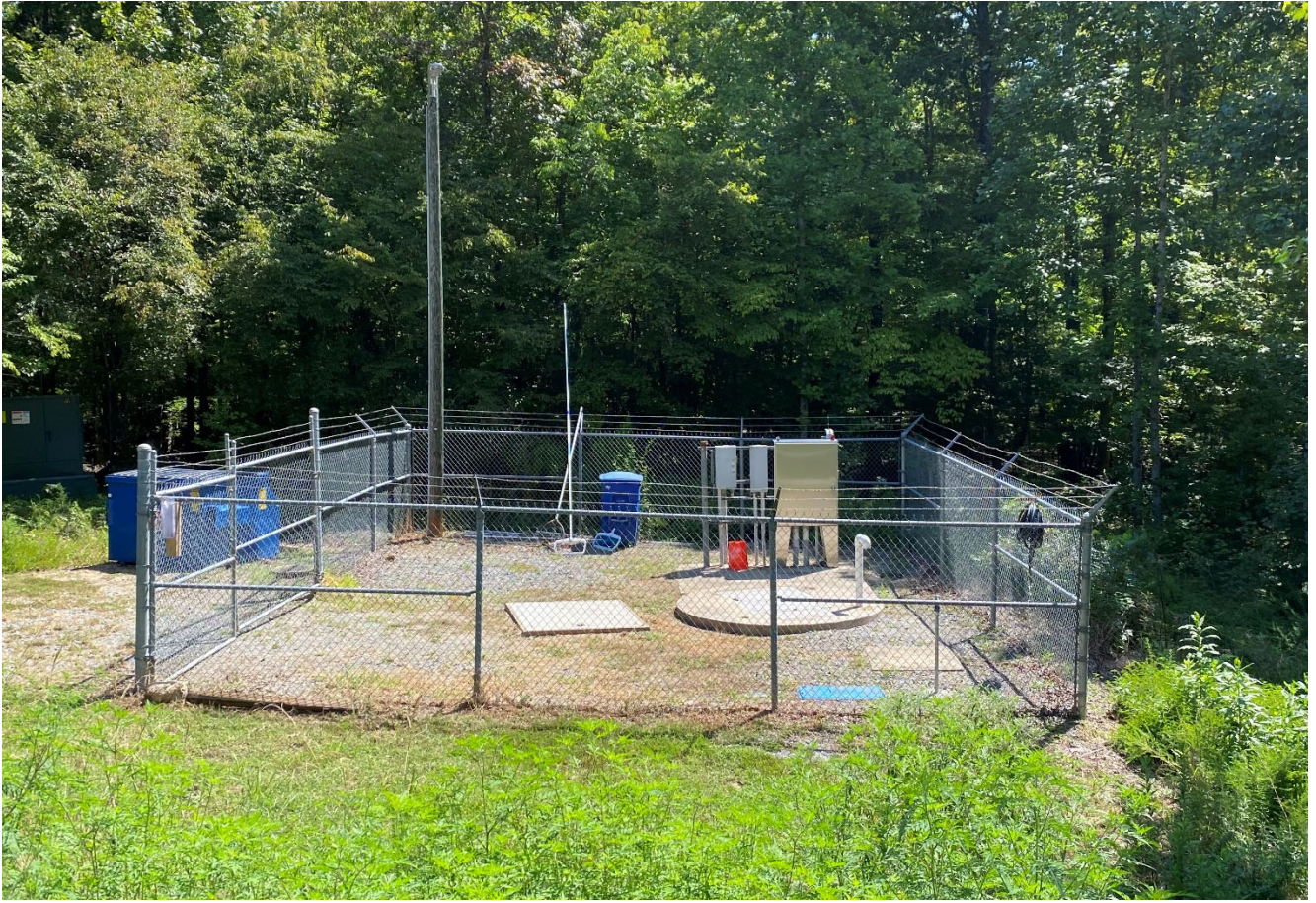
Sturgis Lift Station
